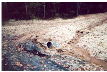
Poorly constructed private access roads can contribute sediment to streams
